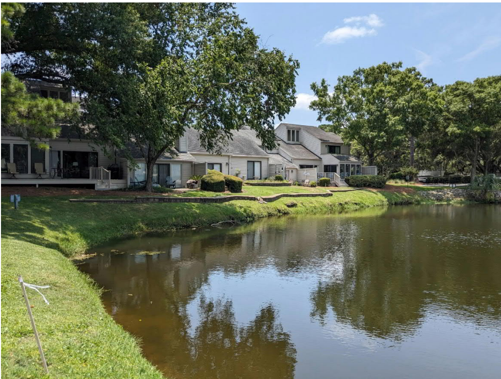
Photo 6: Slope behind Villas 191-195
