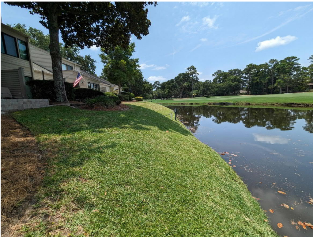
Photo 4: Slope behind Villas 186-190
