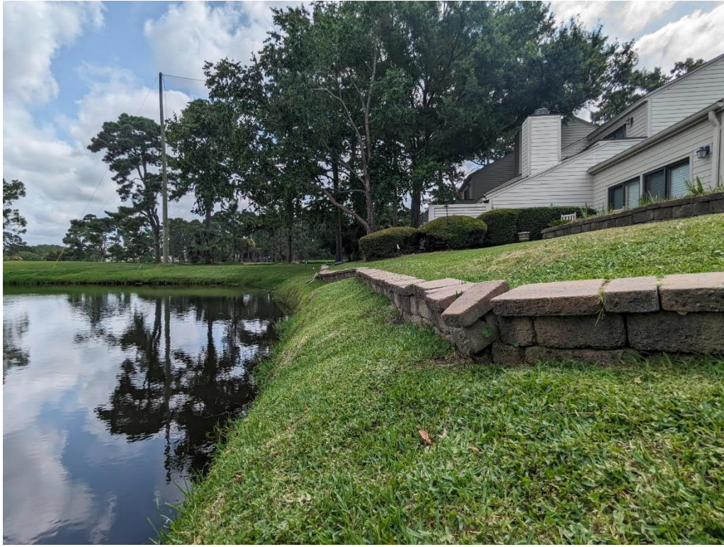
Photo 7: Slope behind Villas 191-195
