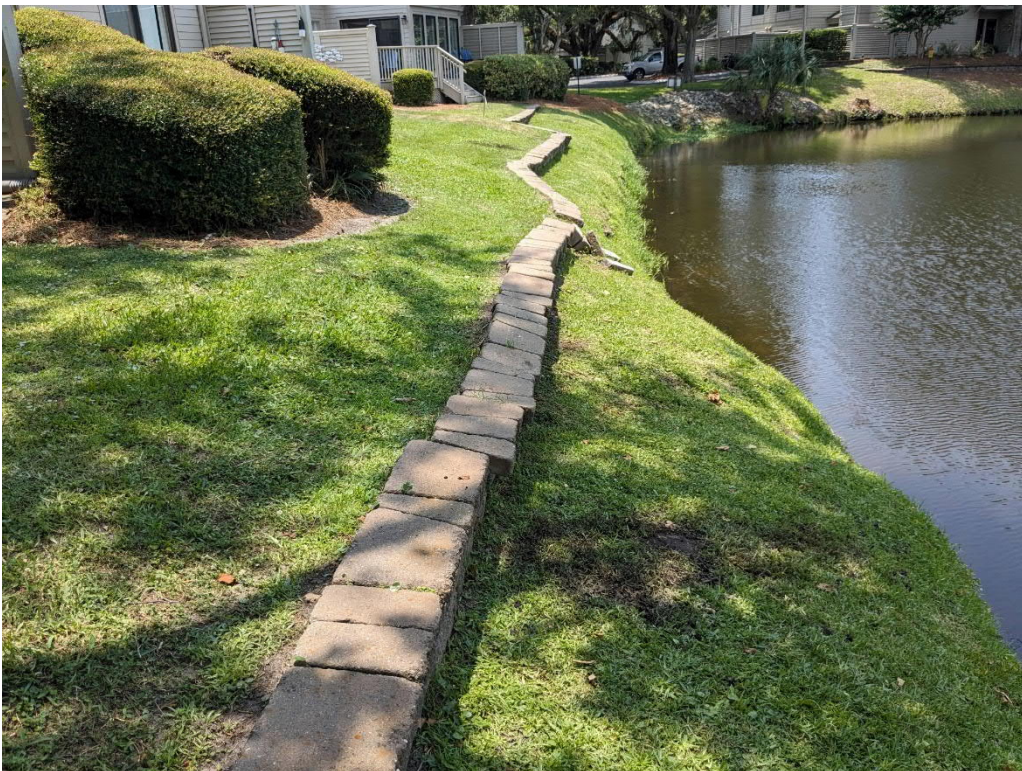
Photo 8: Slope behind Villas 191-195
